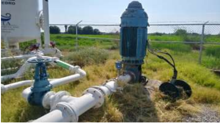
Brackish water well
